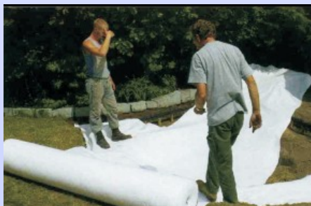
After excavating the soil, first line the hole with fleece, to protect against root & rock penetration.
